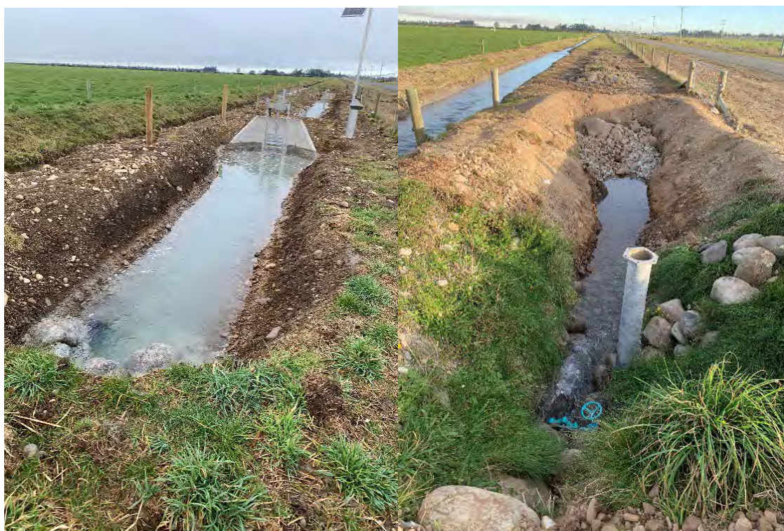
Figure 3-4: MAR 12, Maronan Ealing Road, up gradient (left) and down gradient (right). MAR test site enhanced with buried slotted pipe (Source: M. Neutze)
