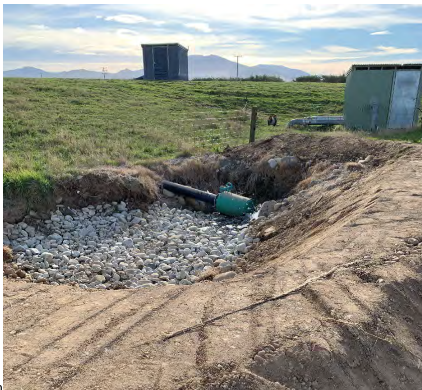
Figure 3-3: MAR 13, Hinds Arundel Road. Enlarged MAR test site (Source: M. Neutze)
