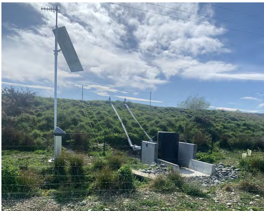
Figure 3-4: MAR09: New intake and flow control infrastructure (Source: M. Neutze)
