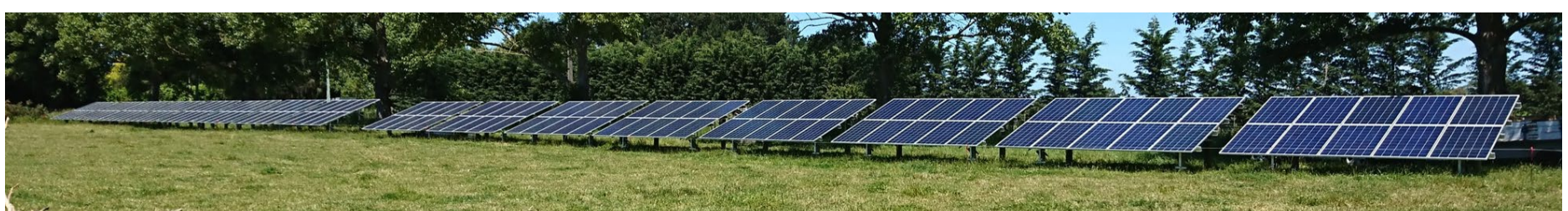
Eiffelton 44 kW Solar Array
